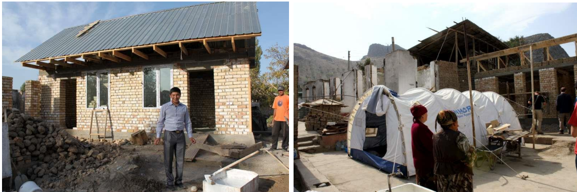
Figure 2.26: Kyrgyzstan shelter by UNHCR (Source: www.unhcr.org )
