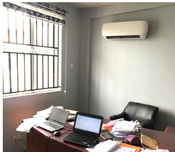
Figure 2.7C Common ventilation system found in the study region.
