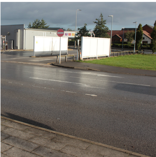
Figure 25 Inconsistent dropped kerbs on Parsonage retail park
